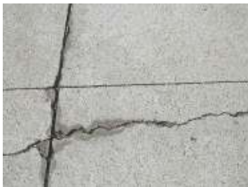
Photo 5 Crack formed outside control joints.
