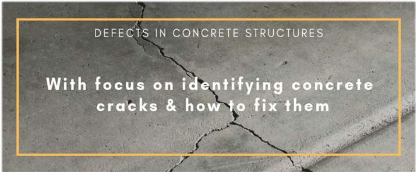
Photo 1 Defects in concrete structures with focus on identifying concrete cracks and how to fix them - Waterstop Solutions
