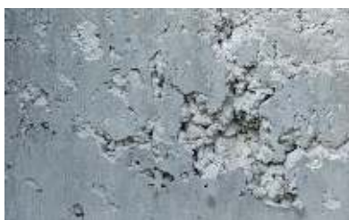
Photo 4 Consolidation related surface issues in concrete.
