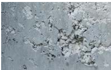
Photo 4 Consolidation related surface issues in concrete.
