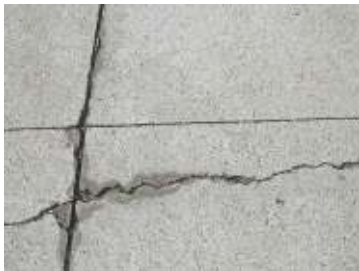
Photo 5 Crack formed outside control joints.
