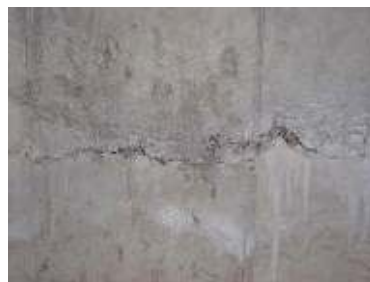
Photo 2 Cold joint - Where old and new concrete do not intermix.
