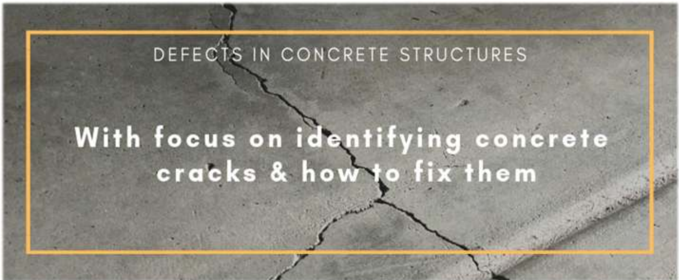
Photo 1 Defects in concrete structures with focus on identifying concrete cracks and how to fix them - Waterstop Solutions
